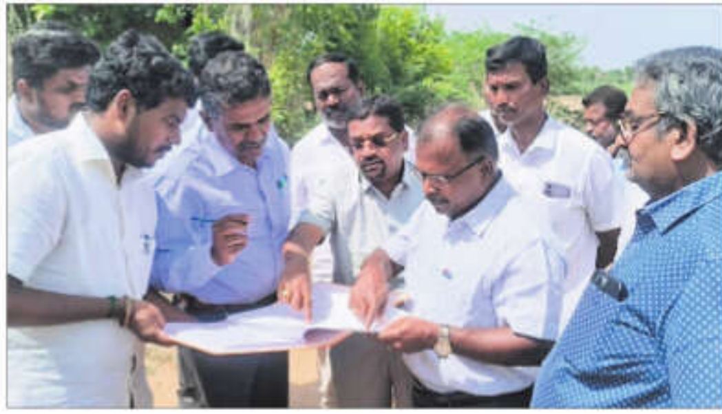
Chief engineer for state highways department Jawahar Muthuraj inspecting the bridge construction site in Karur across the Amaravathi river on Tuesday | EXPRESS
